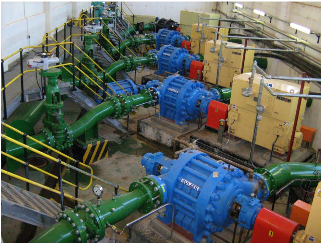
High Lift Pump Station, Five multi-stage pumps (65MI/Day at 351m head)
