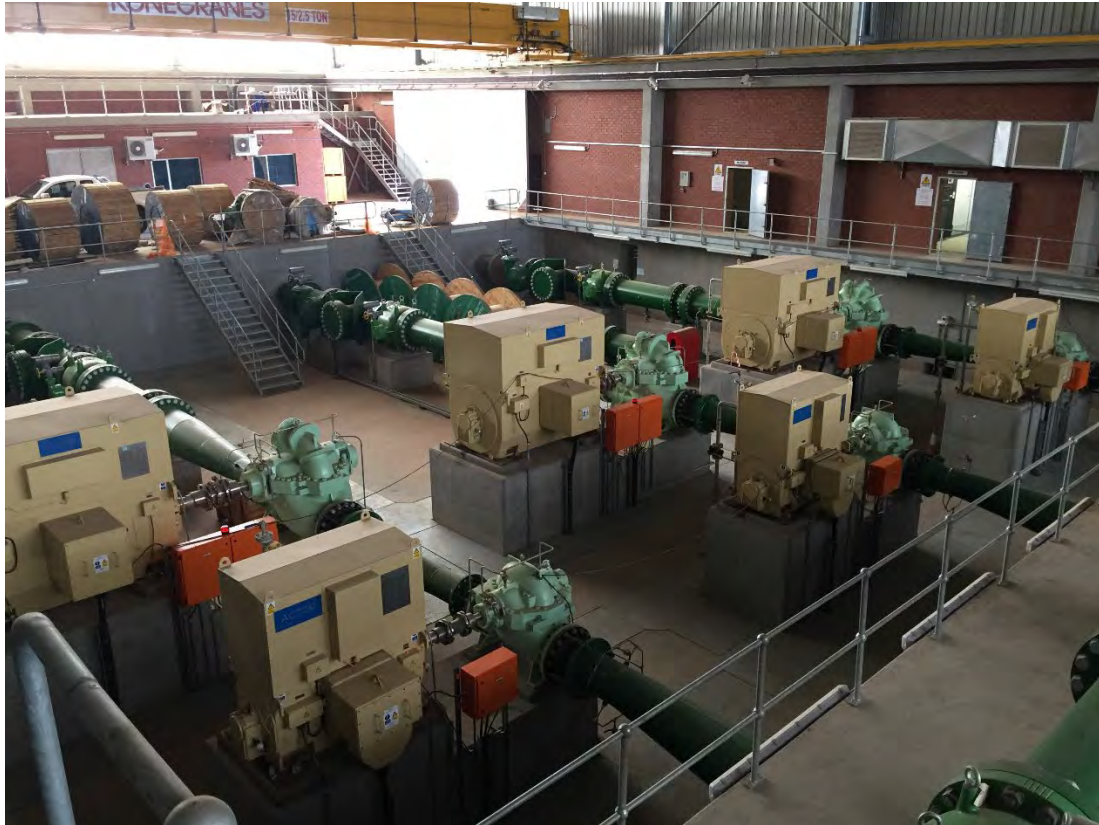
Steelpoort High Lift Pump Station (150MI/Day at 326m head)
