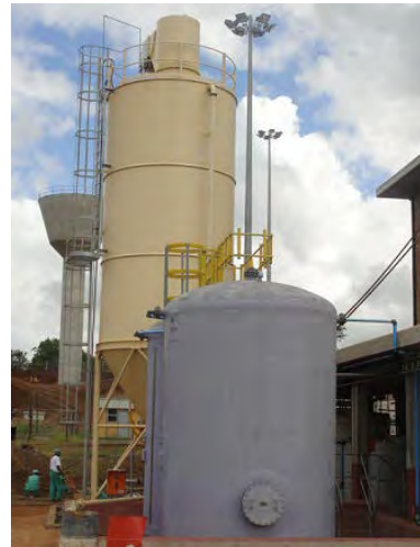
Lime Silo/Chemical Tanks
