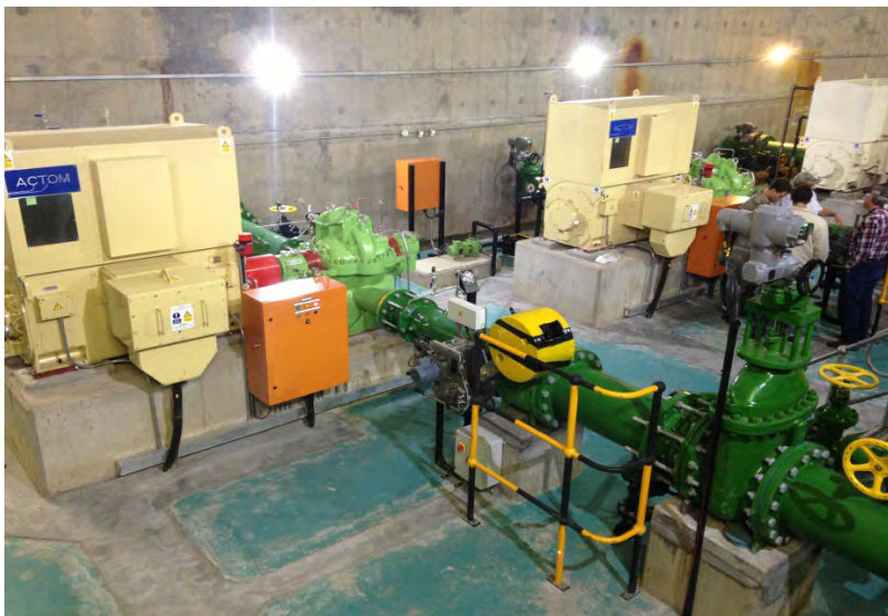
Raw Water Pump Station (1 of 4 lines) 124MI/Day at 130m head
