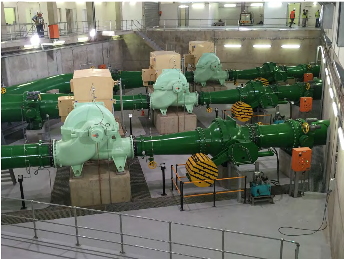
Spring Grove Dam Pump Station (389MI/Day at 67.5m head)
