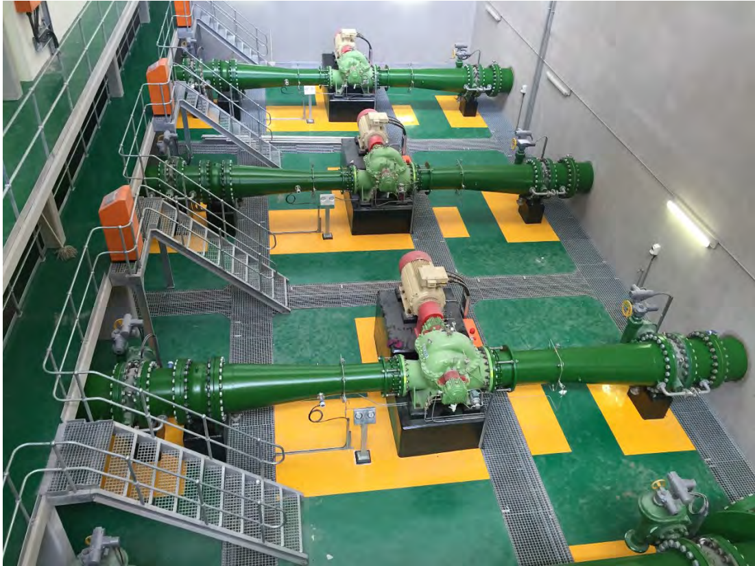
Mokolo Booster Pump Station (109MI/Day)
