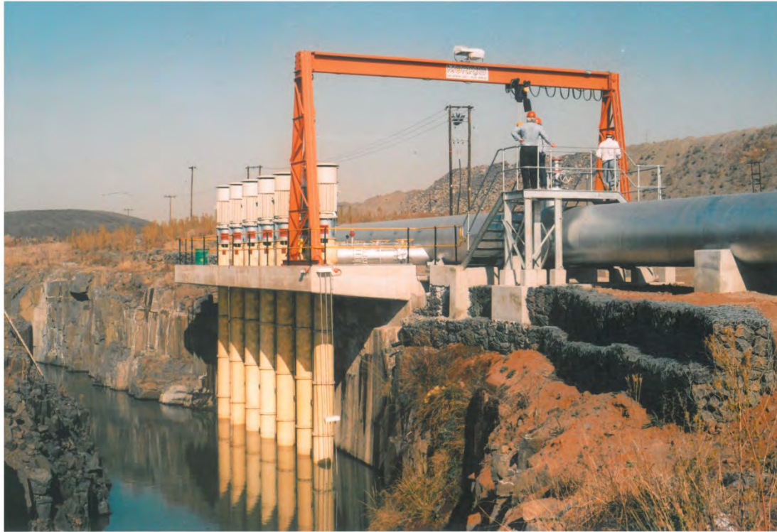
Tweedraaispruit Stream Diversion Pump Station – (Total Output 5.1m 3 /s)
