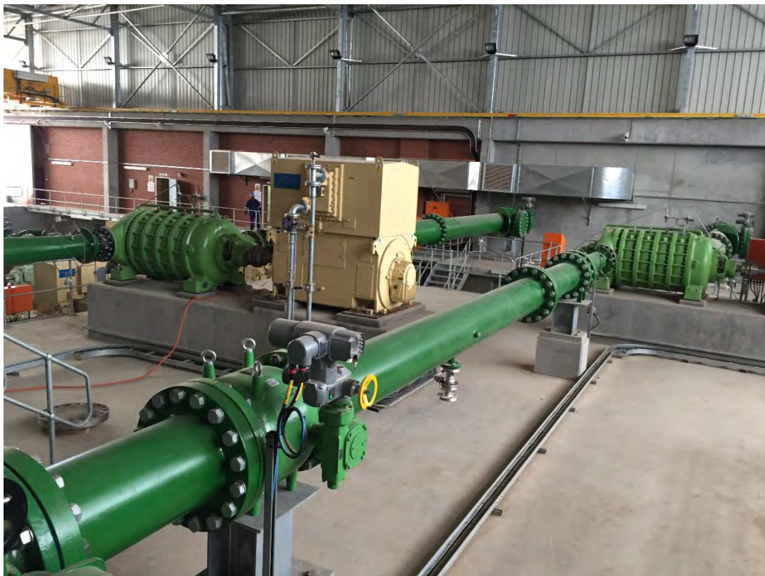
Lebalelo High Lift Pump Station (25MI/Day at 365m head)
