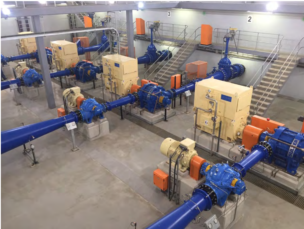
Vaalkop Pump Station (84MI/Day at 306m head)
