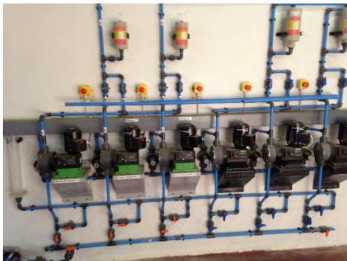
Chemical Dosing Installation
