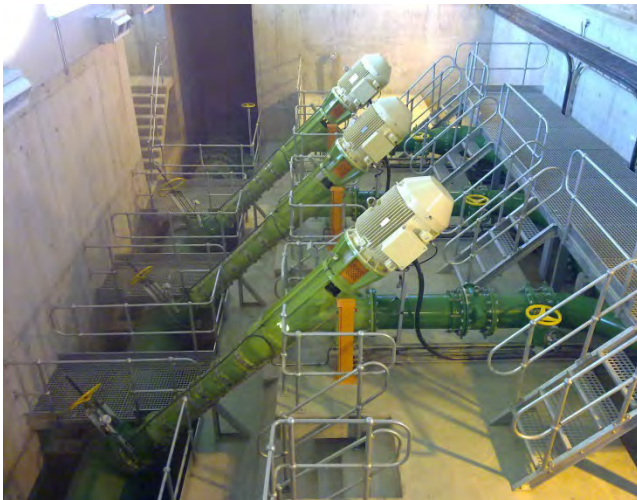
Raw Water Pump Station
