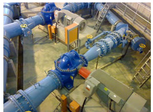
High Lift Pump Station
