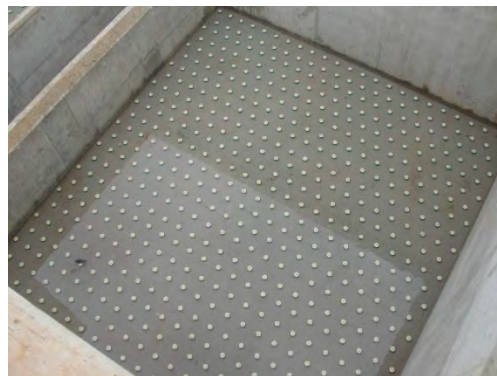
Filter Floor (1 of 32)
